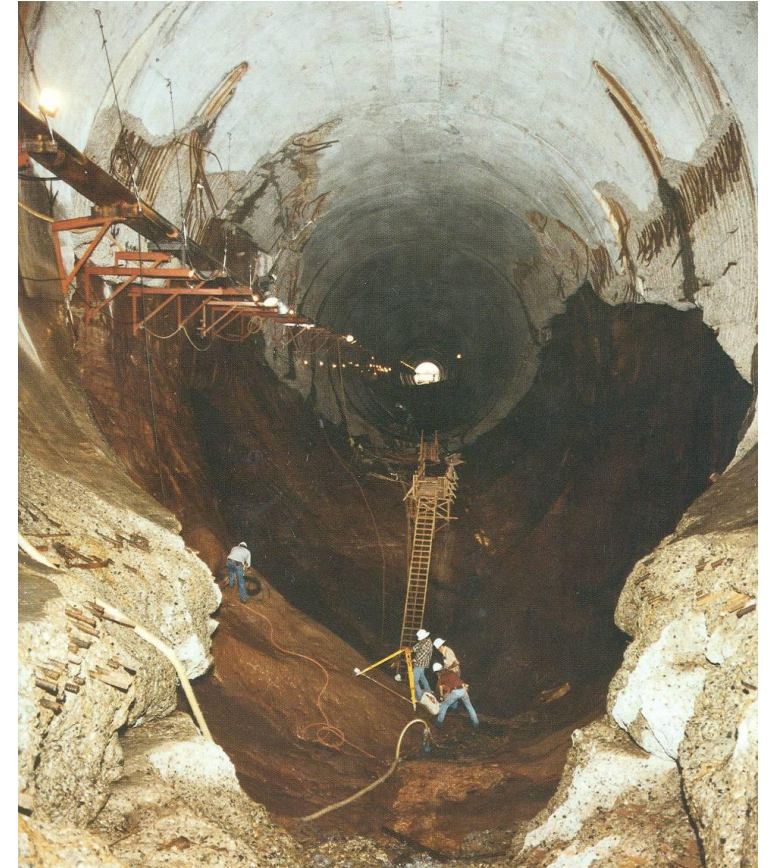
Damaged spillway tunnel at Glen Canyon Dam, 1983. http://geotripper.blogspot.com/2017/02/liveblogging-deluge-concerns-panic-at.html
