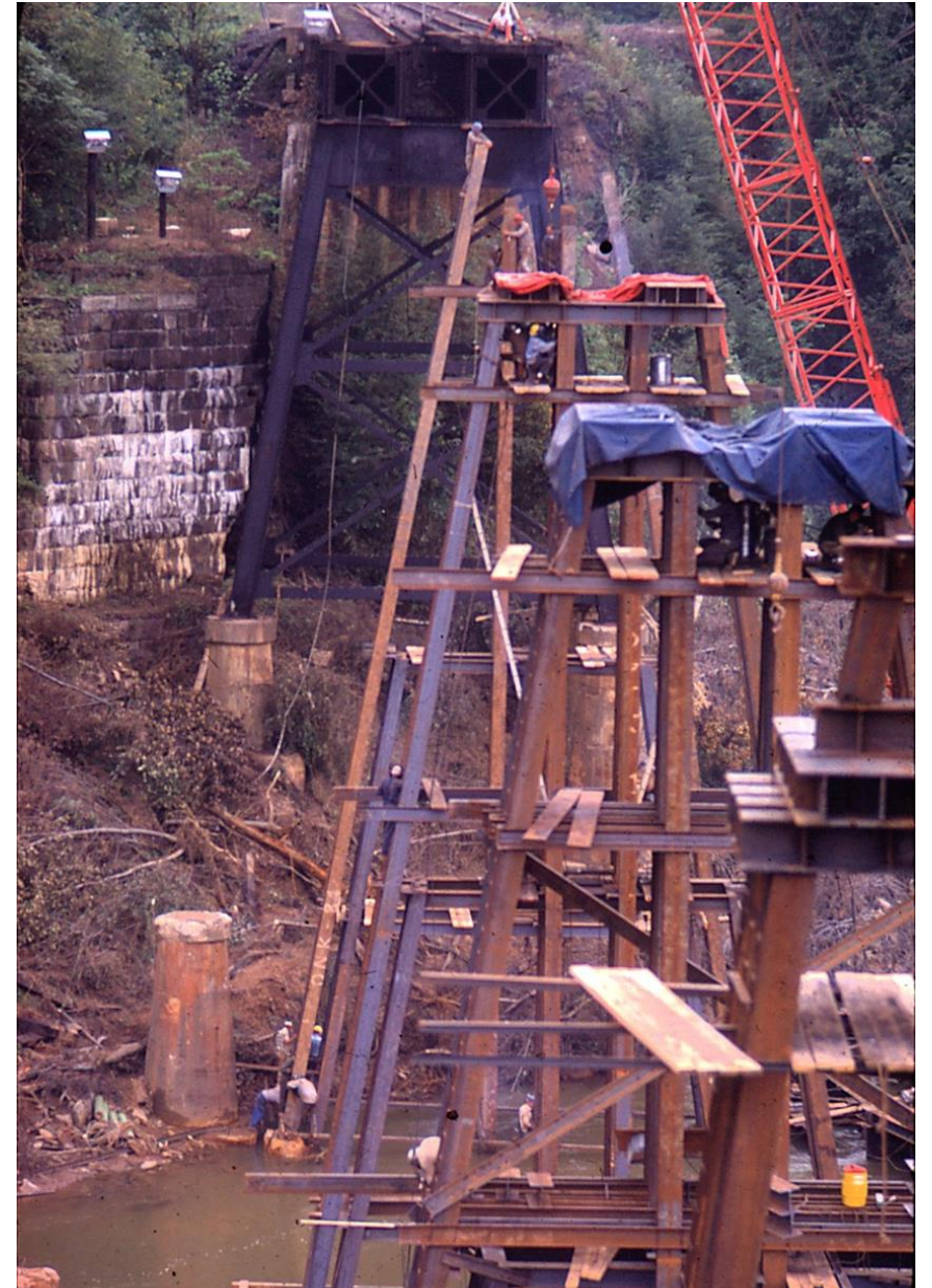
Tower bents under construction. Notice that caps are in place for the bent in the right foreground ready eventually to receive spans
